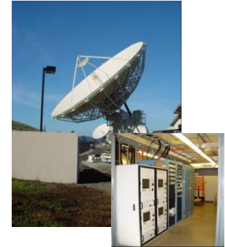
6 Ground Earth Stations
