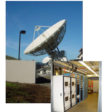
4 Ground Earth Stations
