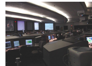
2 Operational Control Centers
