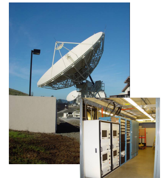
4 Ground Earth Stations
