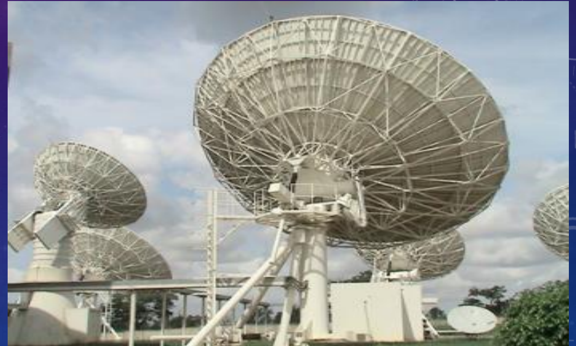
NIGCOMSAT Master Control Station with C-L Band Antenna Systems
