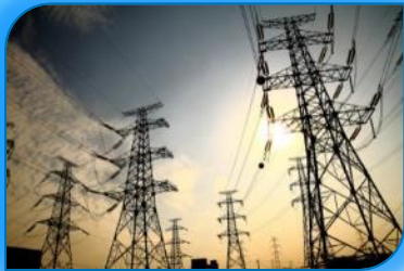
Power Grid Systems
