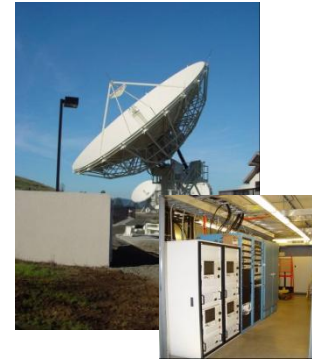
6 Ground Earth Stations
