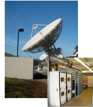
4 Ground Earth Stations
