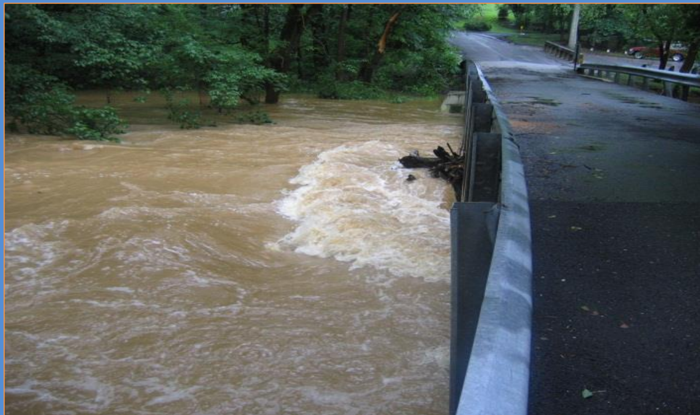
Floating Debris Lodged in a Bridge during Flood Event at Seneca Creek in Germantown, MD
