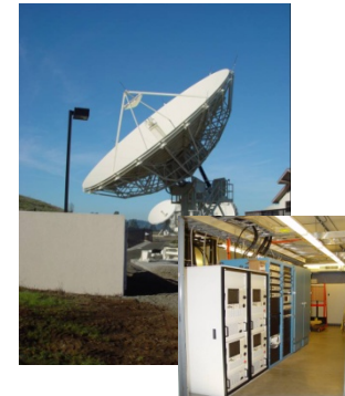
4 Ground Earth Stations
