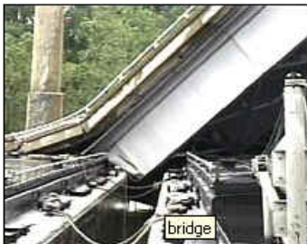
A portion of the I-40 bridge where the barge struck it
