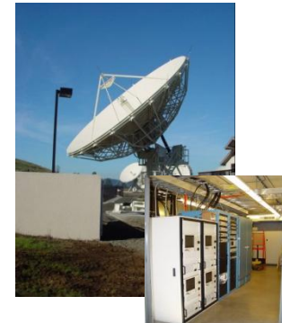
6 Ground Earth Stations
