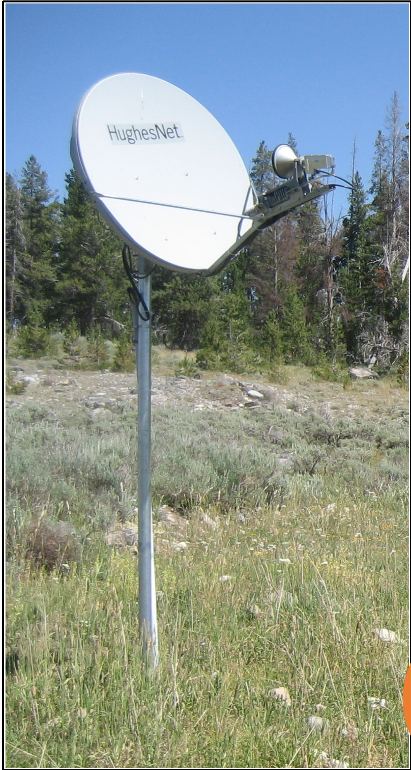
Very Small Aperture Terminal (VSAT)
